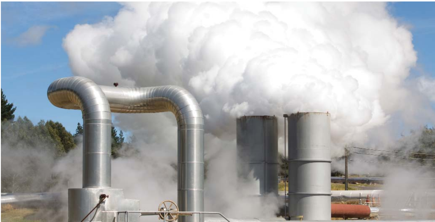
Geothermal power station.
